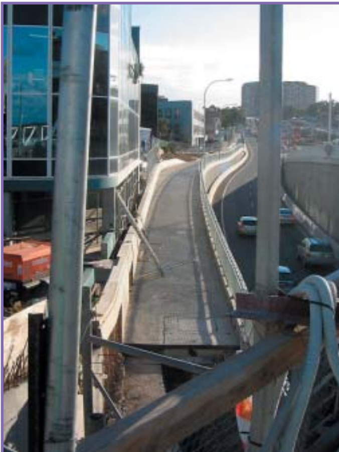
alongside Gore Hill Freeway looking west of Reserve Rd. Artarmon... foreground is part of the $4million underpass of Reserve Rd
