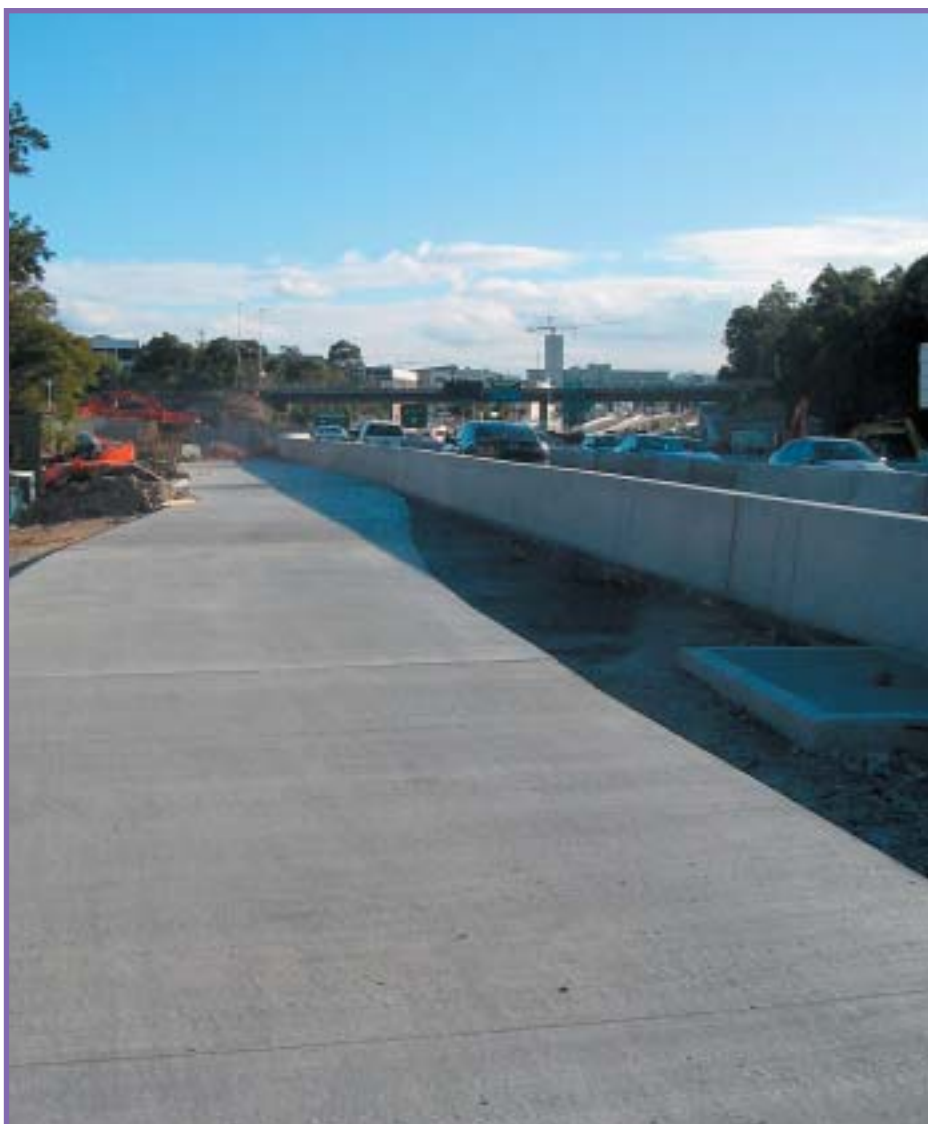
alongside Gore Hill Freeway just west of the railway line, near Punch St, Artarmon
